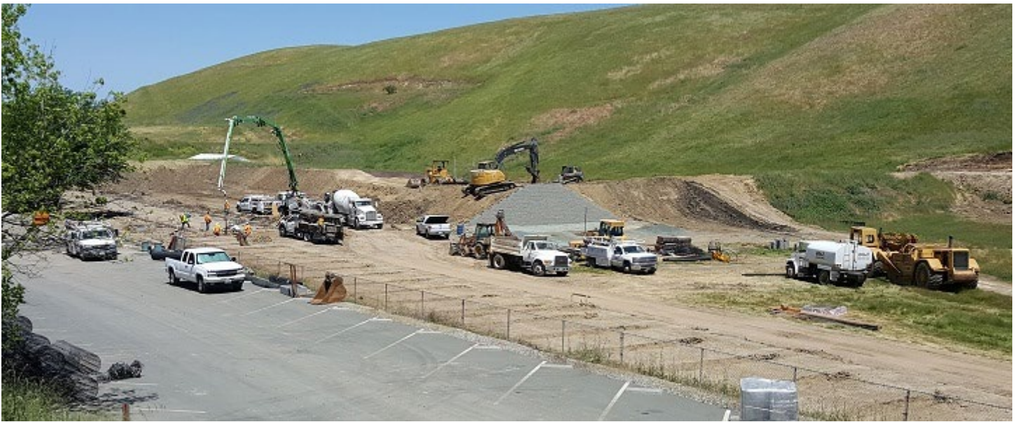
May 2 first concrete pour on Pistol Range, pistol berm wall up between pistol & rifle
